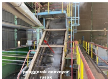
Gambar 6 Fasilitas Dewatering Mill Feed Conveyor
