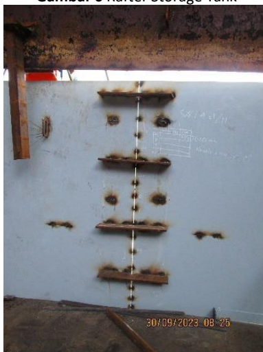
Gambar 6 Rafter Storage Tank
