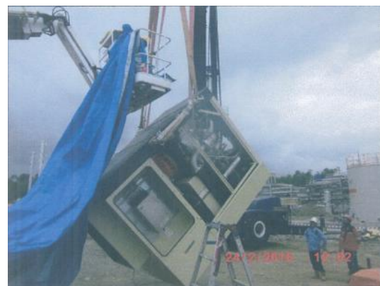
Gambar 5. Posisi Air Compressor B ((373-V-1001B) Twisted
