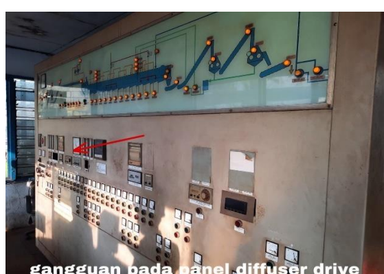
Gambar 7 Panel Diffuser Drive
