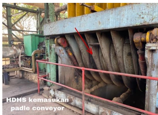
Gambar 10 Fasilitas Heavy Duty Hammer Shredder (HDHS)
