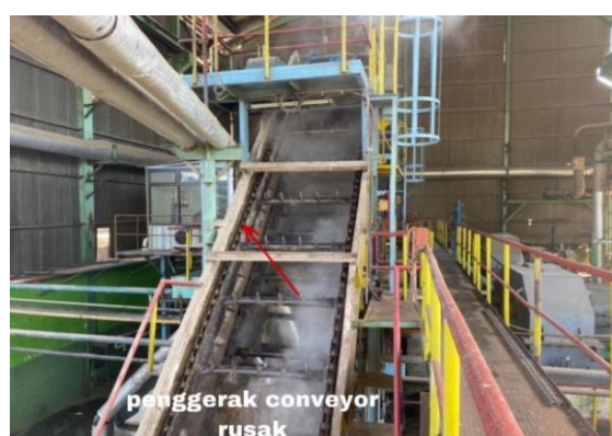
Gambar 6 Fasilitas Dewatering Mill Feed Conveyor
